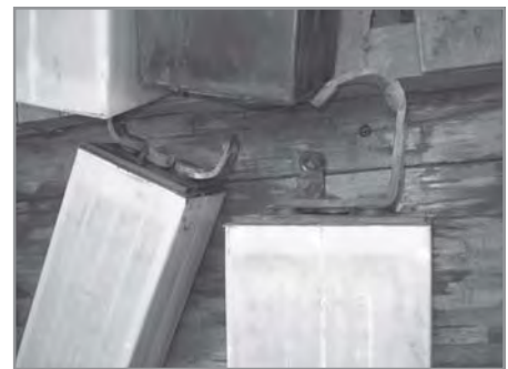
Picture 1: Batteries on side and leaking acid in trailer
